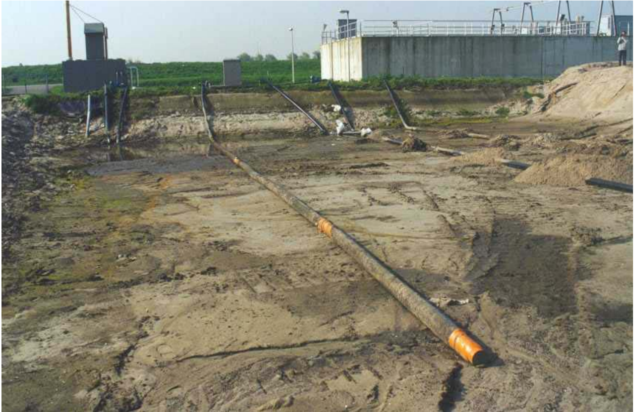
Figure 2. Drainage system at pilot Nauerna
